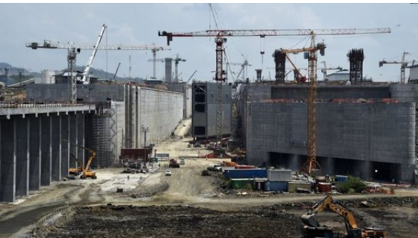
Image copyright Getty Images Image caption The new lock gates on the Panama Canal weigh up to 700 tonnes and measure almost 30 metres high
