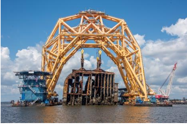
The VB-10000 hoists the final section of the Golden Ray wreck, Section Four, slowly out of St. Simons Sound on Saturday, October 16, 2021. St. Simons Sound Incident response photo.
